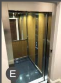
E Electric 230 volt lift (8 person)
