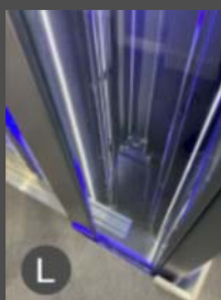
L Led Lighting throughout entire lift shaft
