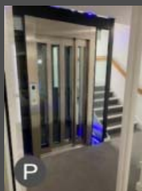
P Passenger Lifts
